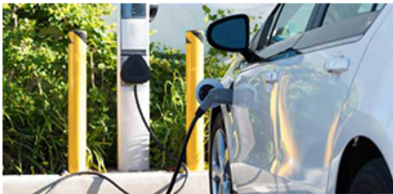
IBEW is continuing a national push to certify and train members to install EV charging infrastructure.
